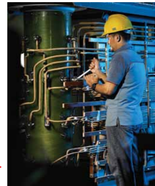
▶ Transformer with on load tap changer. Trafo dengan on load tap changer.
